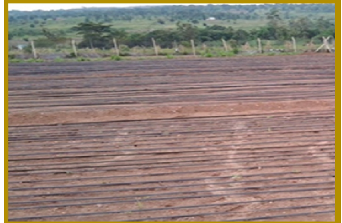
The CFT site in Uganda: up is the seed store, office and drying platform and below is the field with fully installed drip irrigation facility
